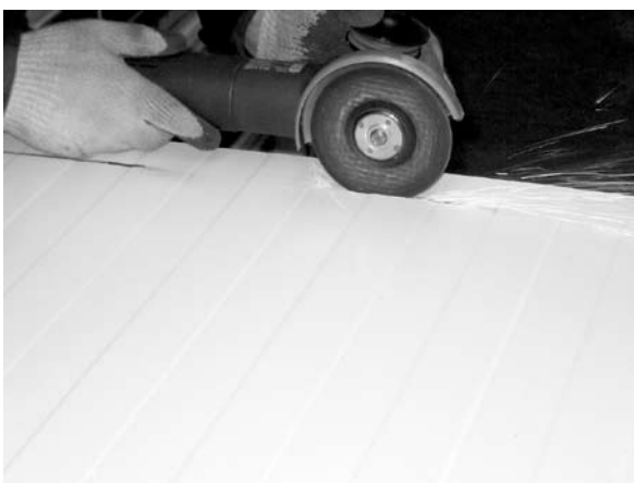
Pic. 2. Do not cut panels with angular grinding machine as anticorrosive covers can be devastated.
